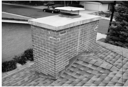
Clay Liner Cover
